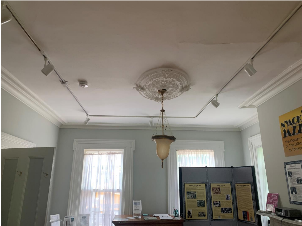
Figure 12. Suite 1A - Cracking at ceiling
