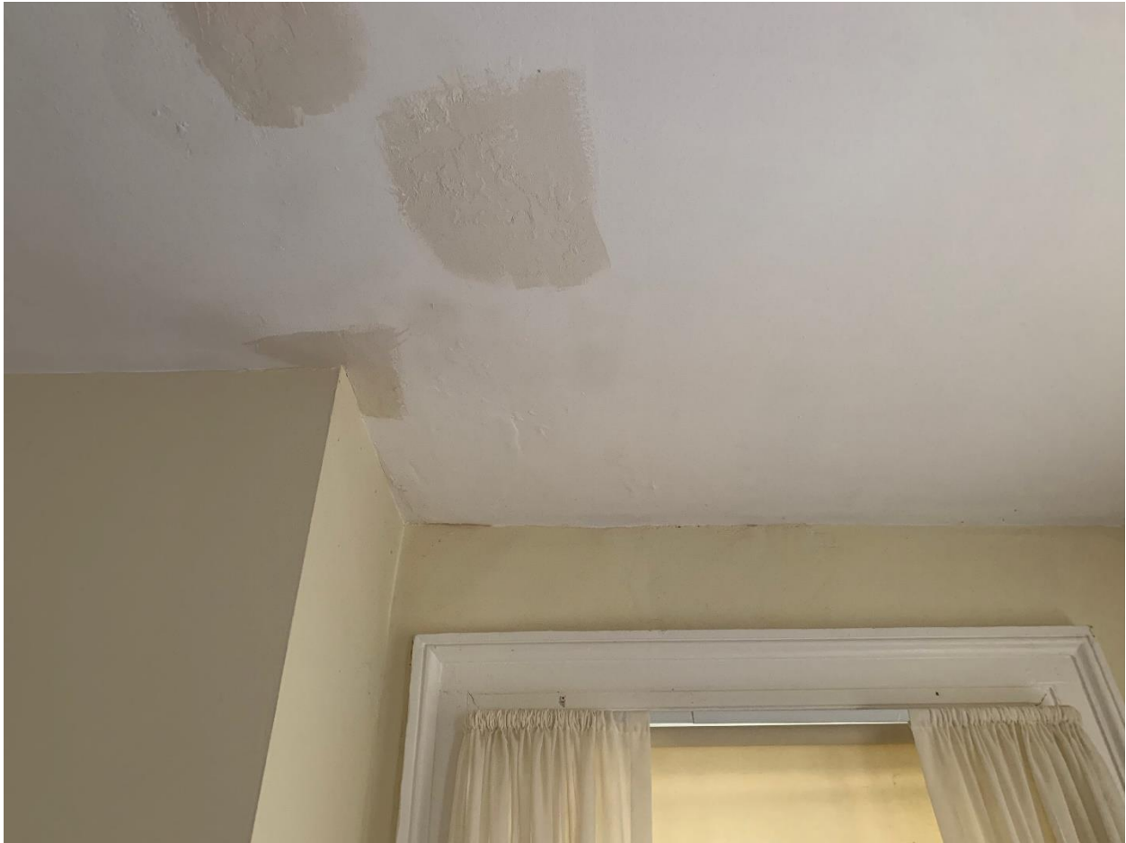
Figure 17. Suite 2B - Water damage and staining at ceiling located at the second level.
