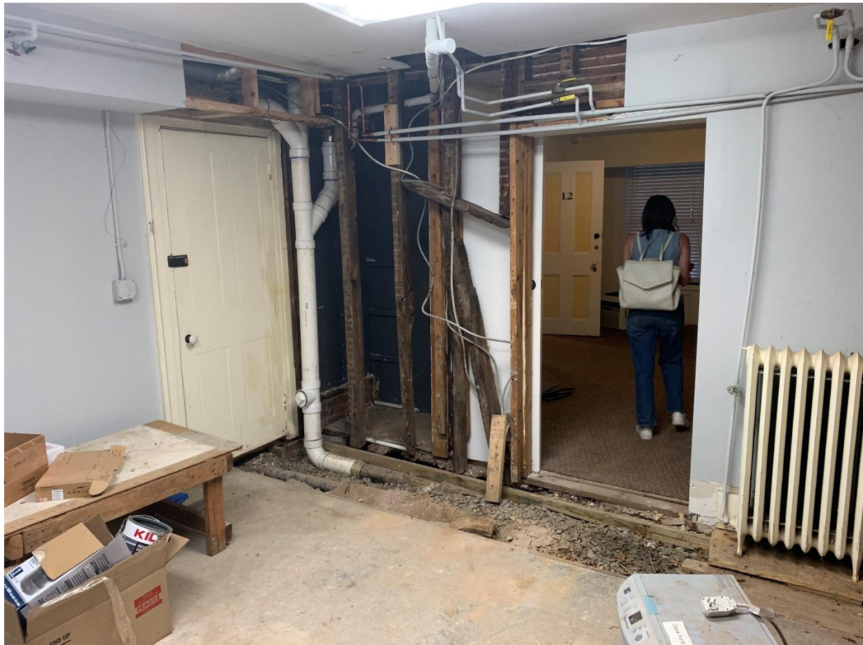
Figure 3. Basement- Condition of interior partition wall adjacent to plumbing work
