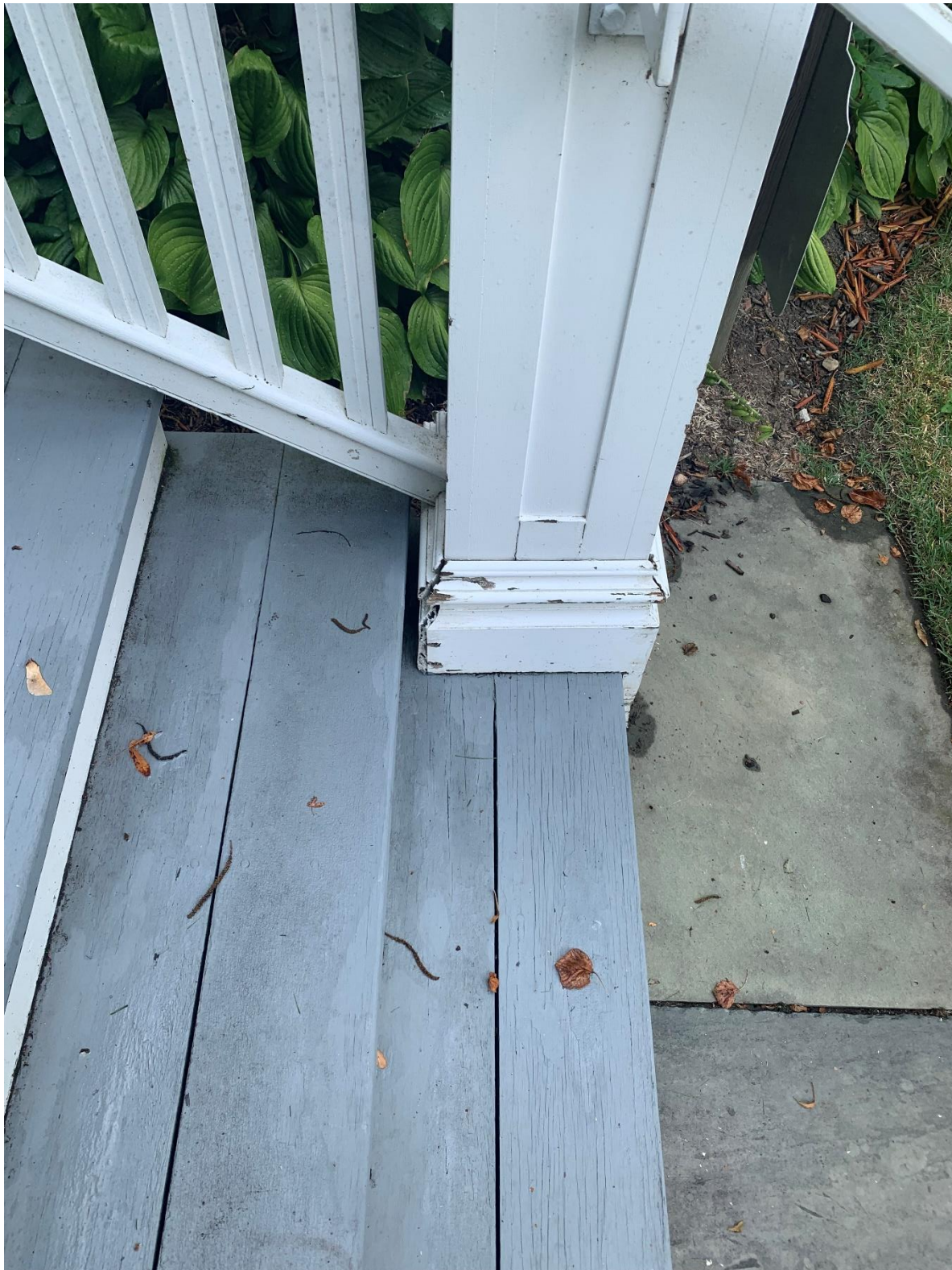
Figure 29. Damaged base molding of handrail post at bottom of stairs of the front entry.
