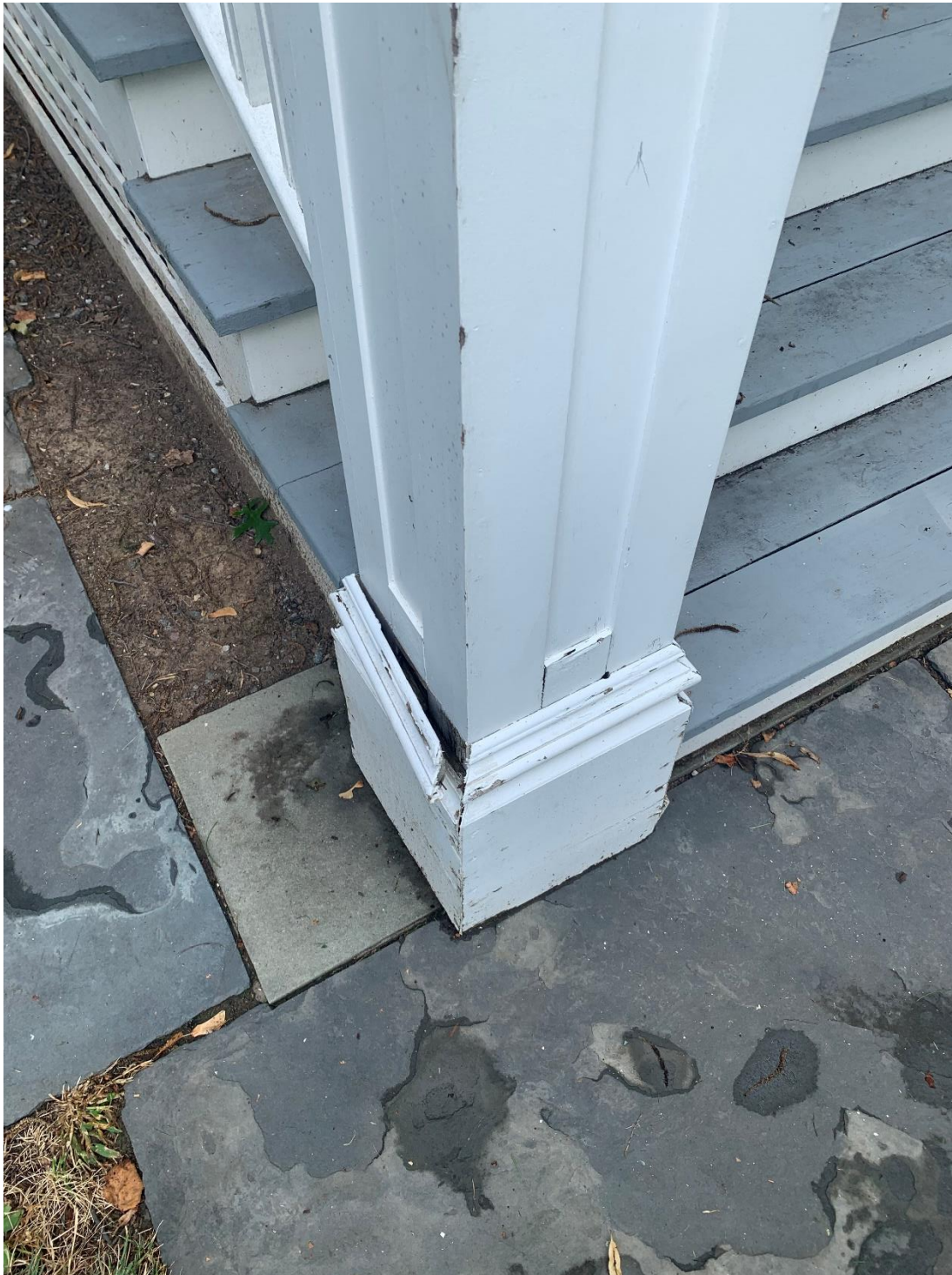
Figure 28. Damaged base molding of handrail post at bottom of stairs of the front entry.
