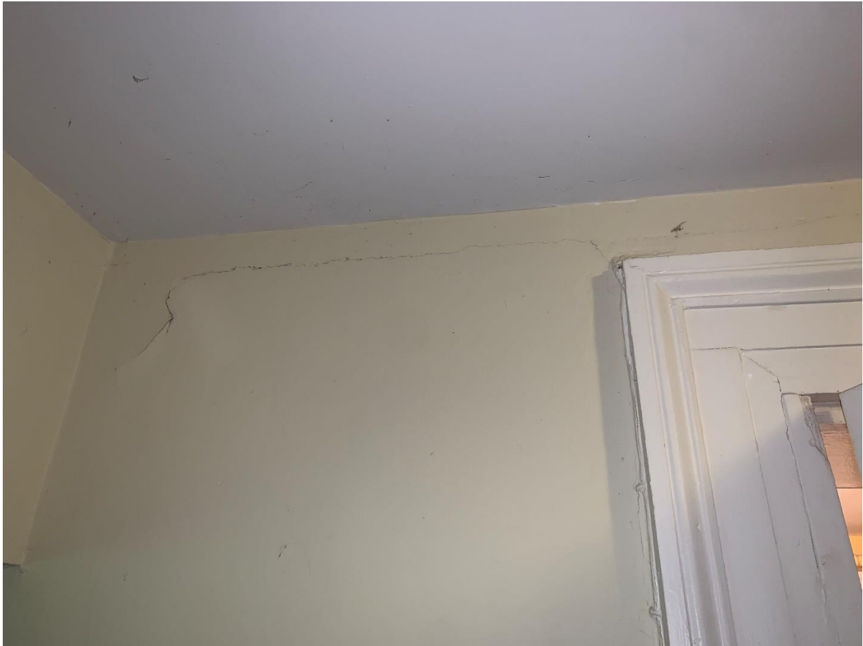
Figure 8. Suite 1B - Cracking at wall starting at the door frame located at the first level.
