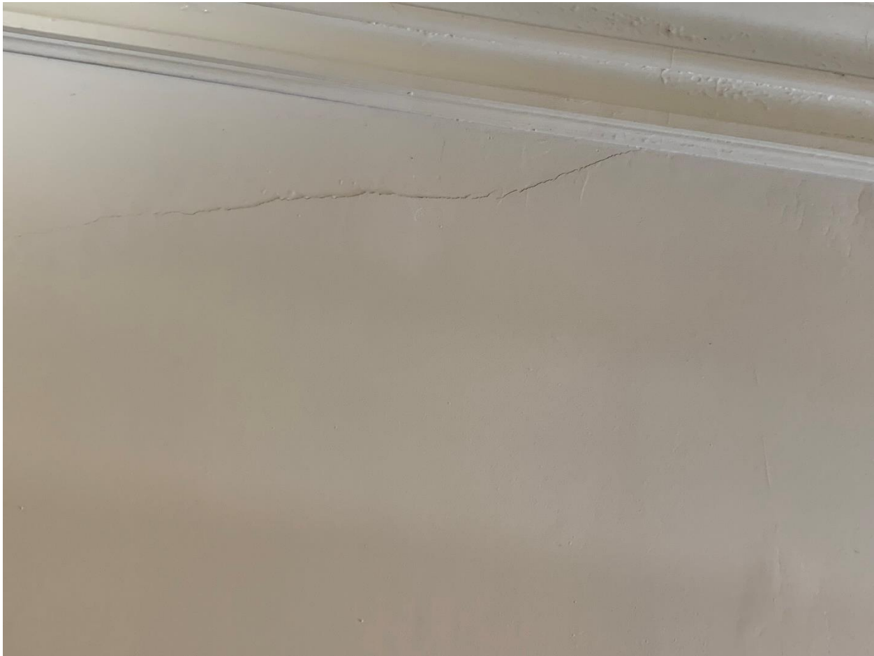
Figure 9. Suite 1B - Cracking at ceiling located at the first level.
