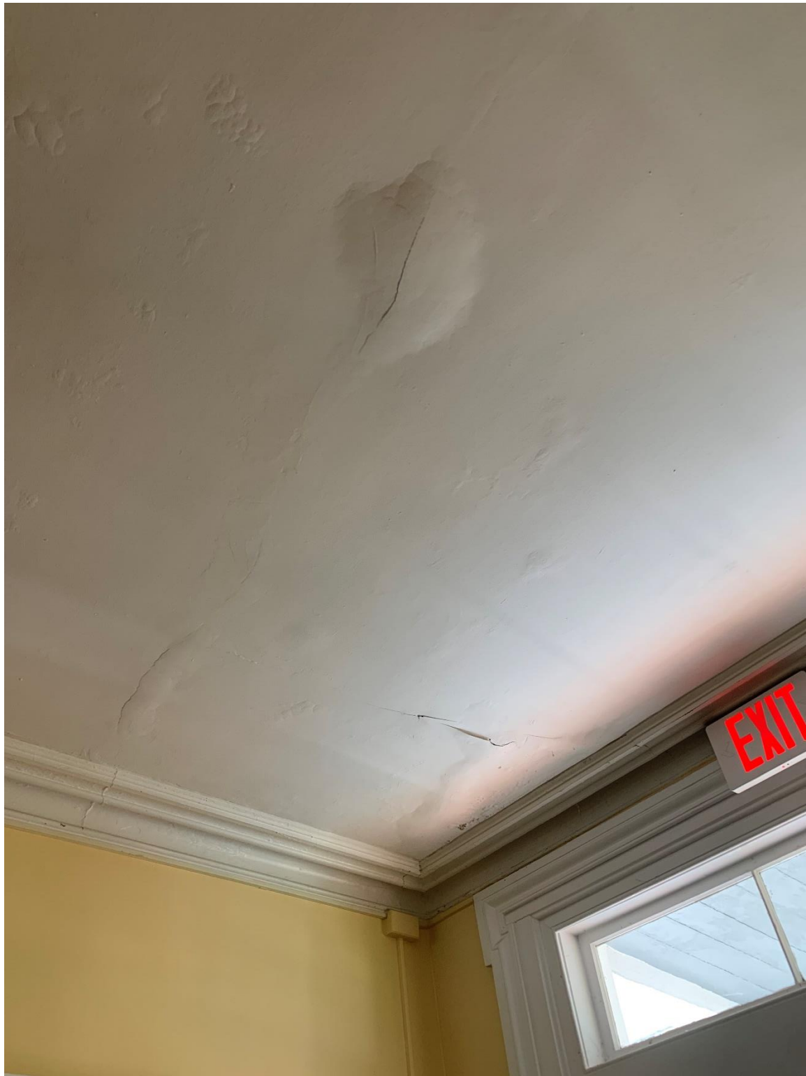
Figure 6. 1 st floor hallway - Ceiling Cracks/Water Damage at 1st Floor Rear Entry
