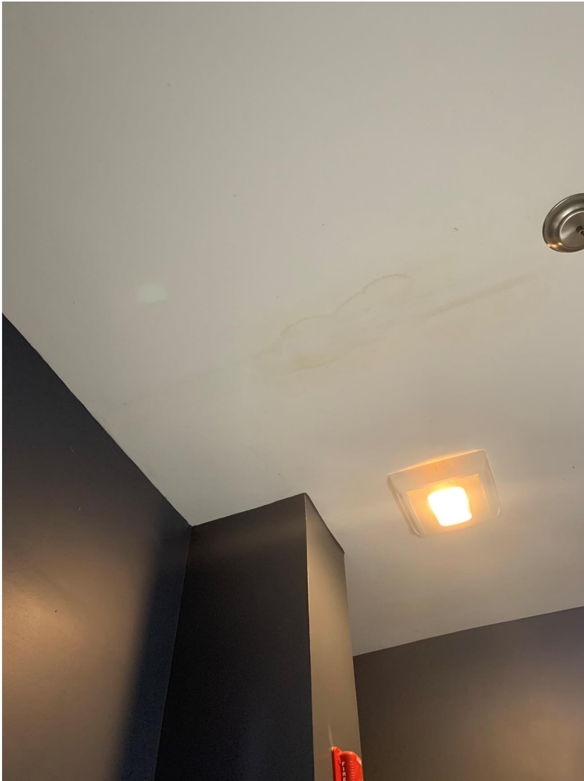
Figure 11. 1 st floor bathroom - Water damage at ceiling
