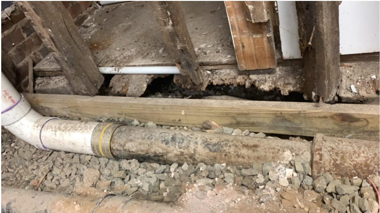
Figure 4. Basement- Condition of base of partition wall
