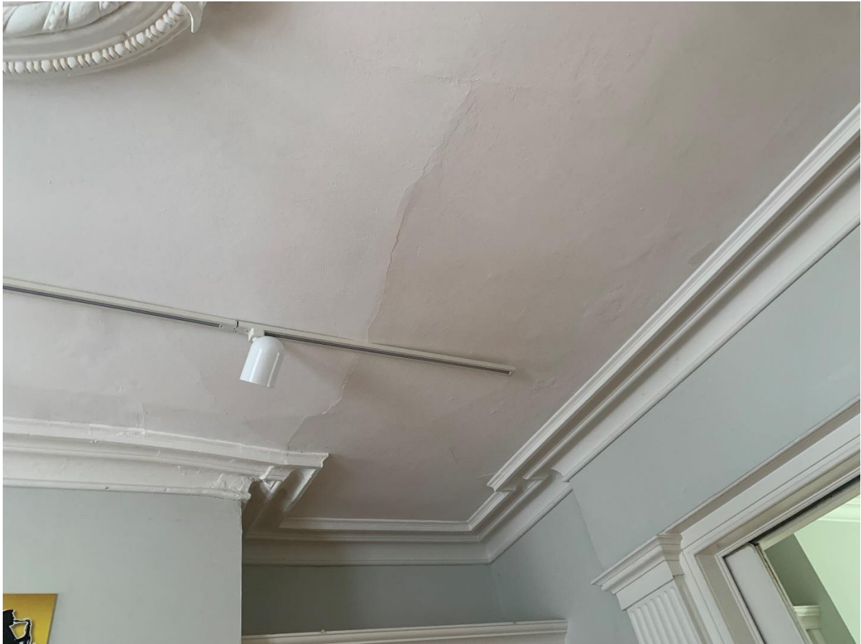
Figure 13. Suite 1A - Cracking/bulging at ceiling
