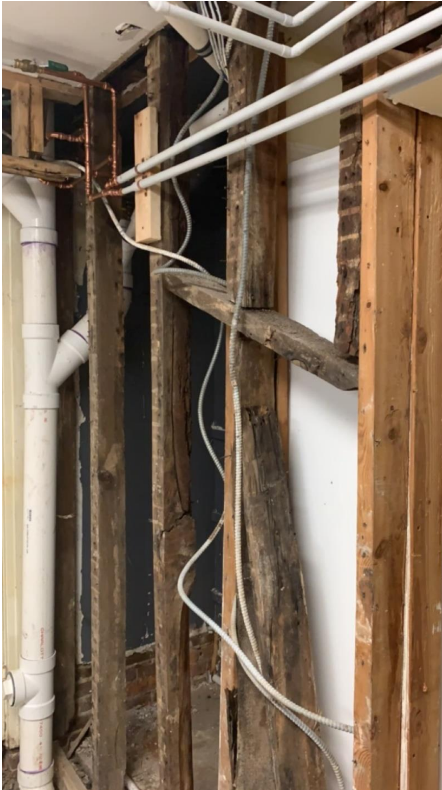
Figure 5. Basement - Condition of exposed stud framing at basement level
