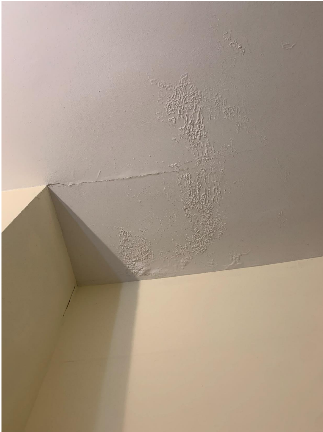
Figure 10. Suite 1B - Water damage at ceiling located at the first level.
