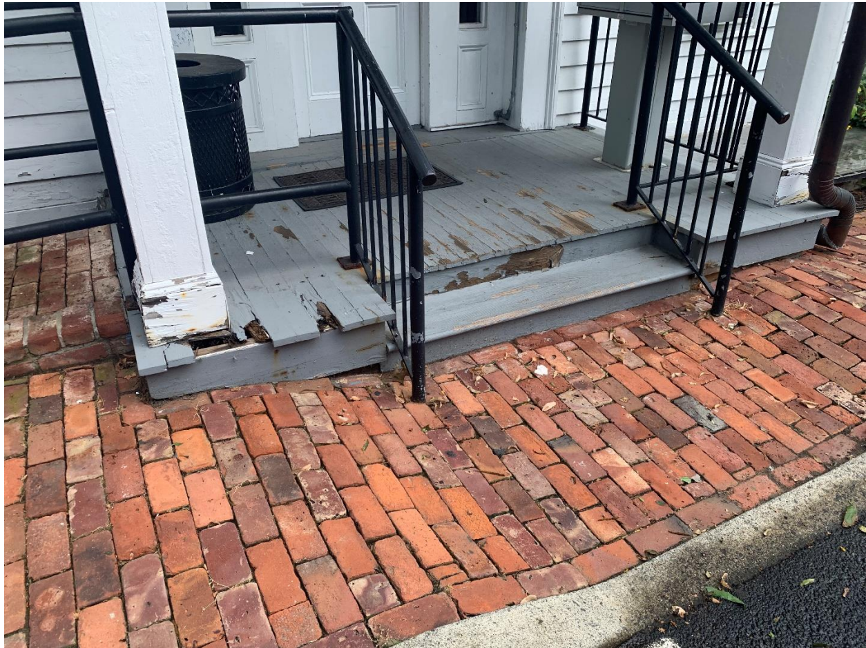
Figure 26. Damaged wood decking at back entry adjacent to parking lot.
