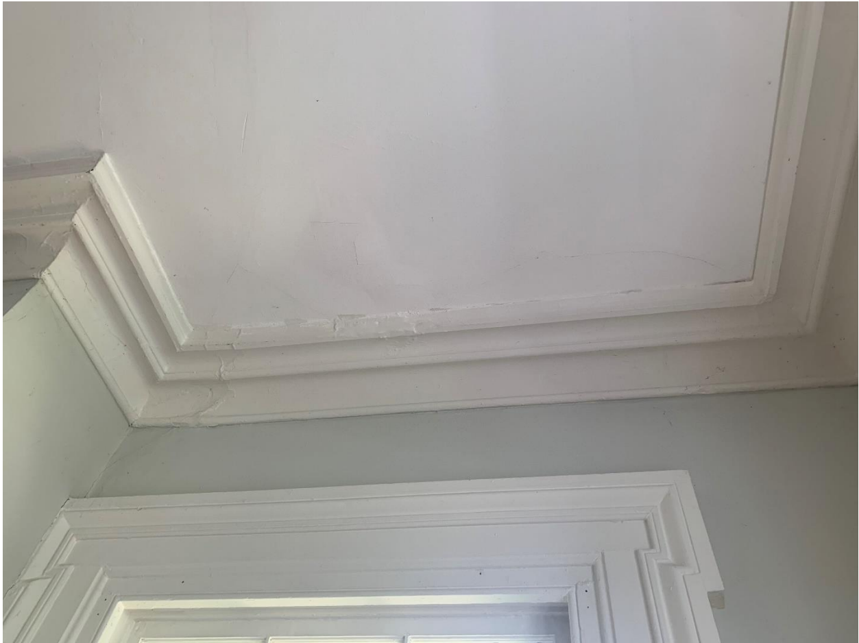
Figure 14. Suite 1A - Apparent water damage and cracking at ceiling located at the first level.
