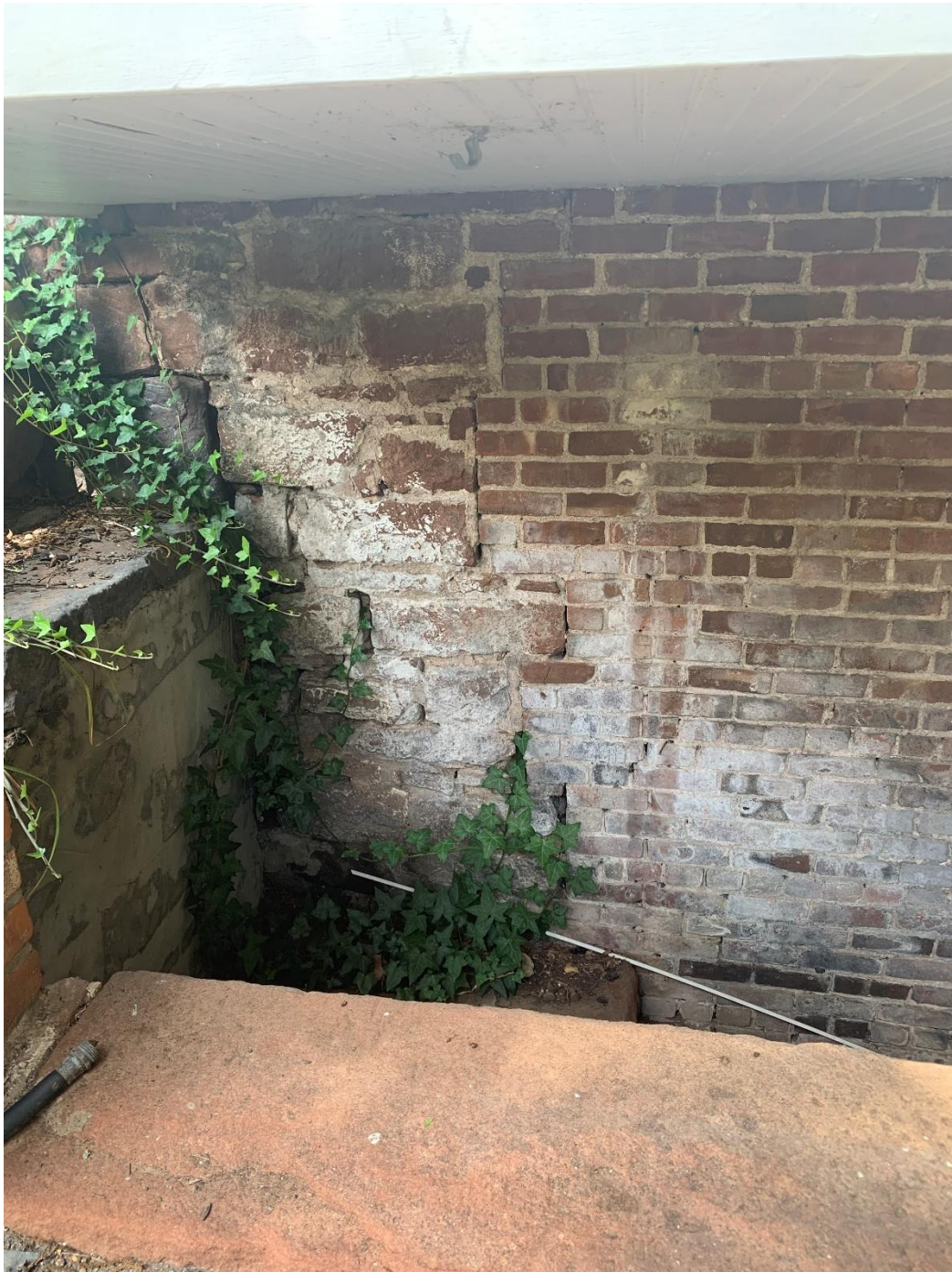
Figure 24. Damaged rubble retaining wall at southwest corner
