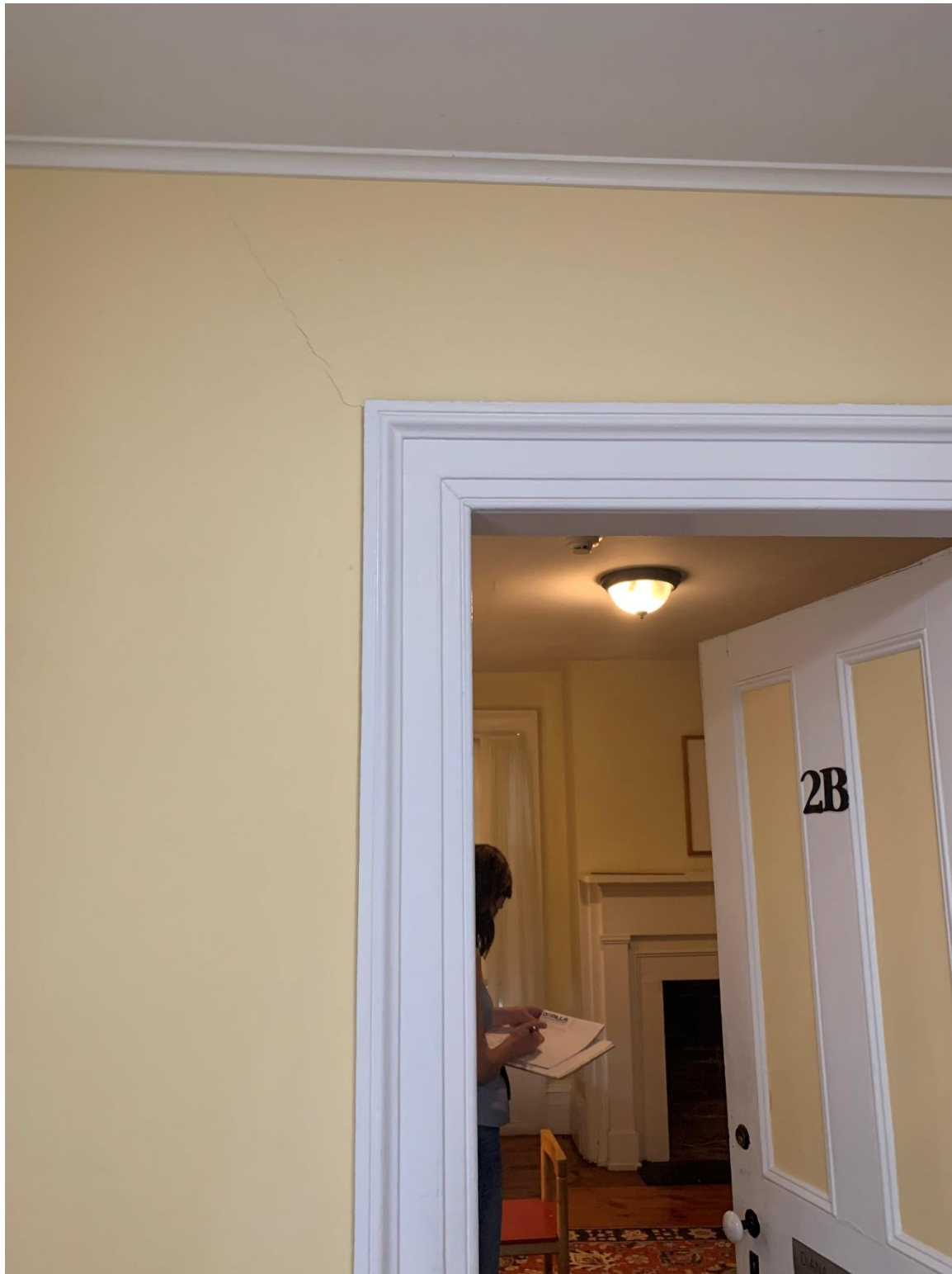
Figure 18. Hallway outside 2B - Cracking at door frame located at the second level.
