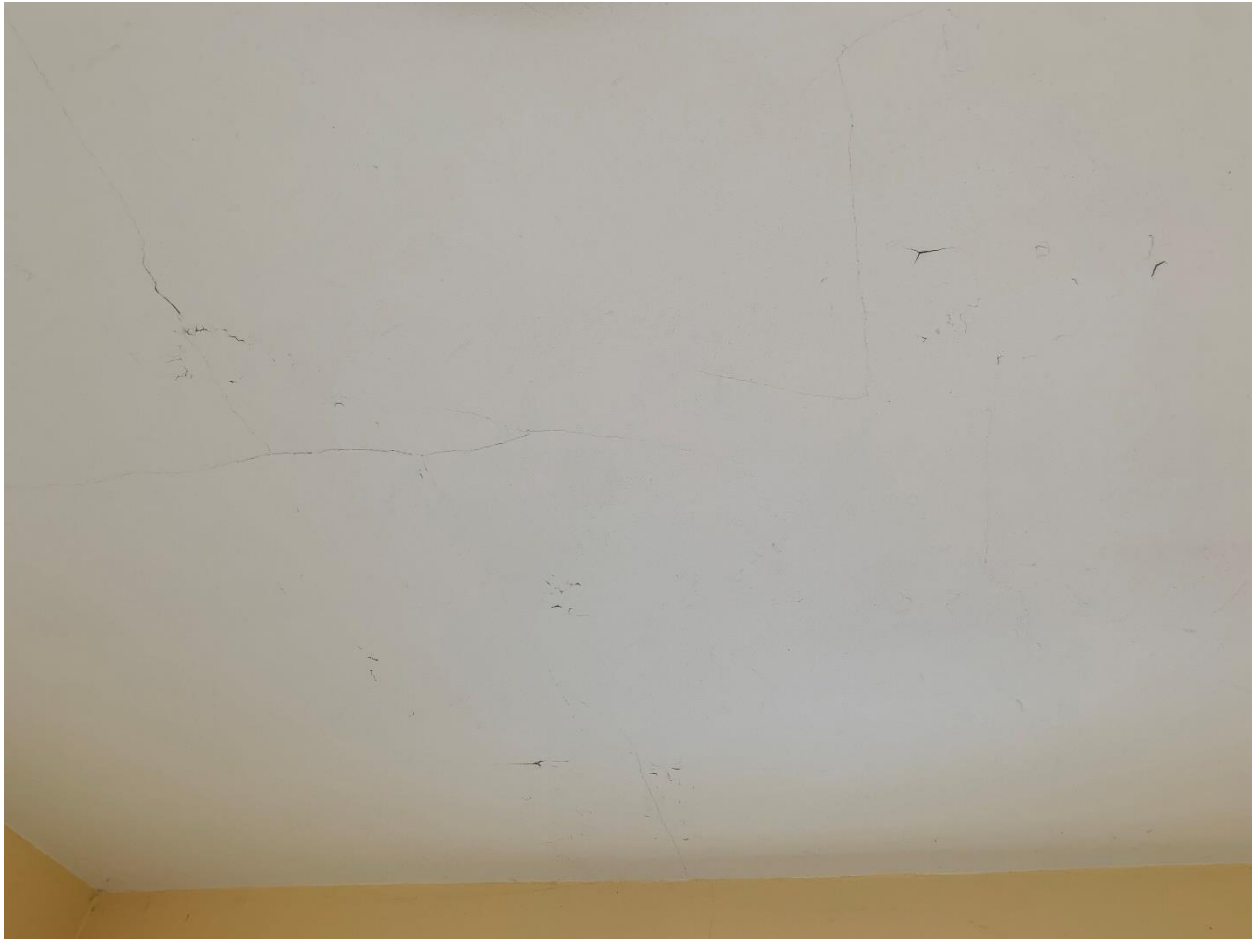
Figure 20. Suite 2D - Cracking at ceiling of 2 nd floor
