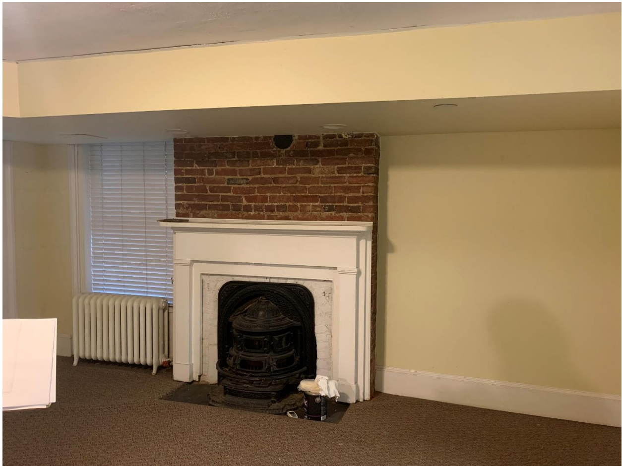
Figure 1. Basement - Drywall separation at ceiling between finishes located at basement level.
