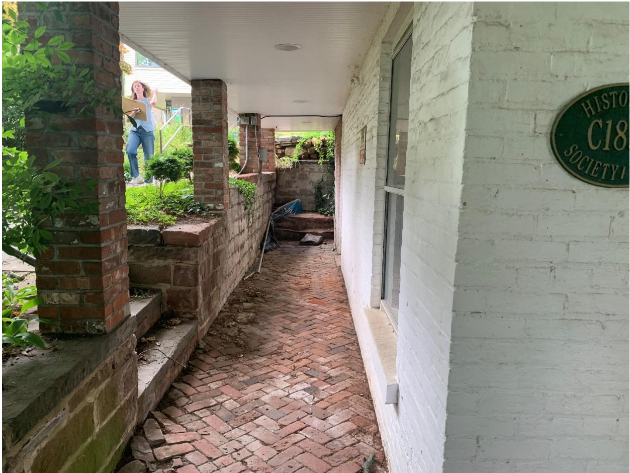
Figure 23. Condition of Pavers at Basement Patio
