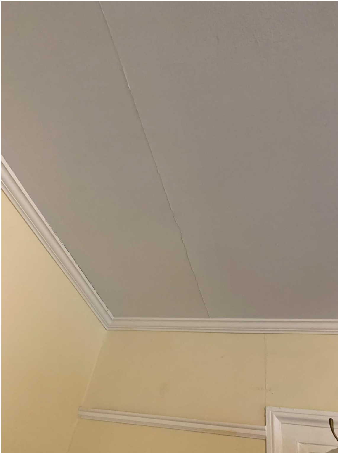
Figure 15. Suite 2B - Cracking of Ceiling Finish at 2nd Floor
