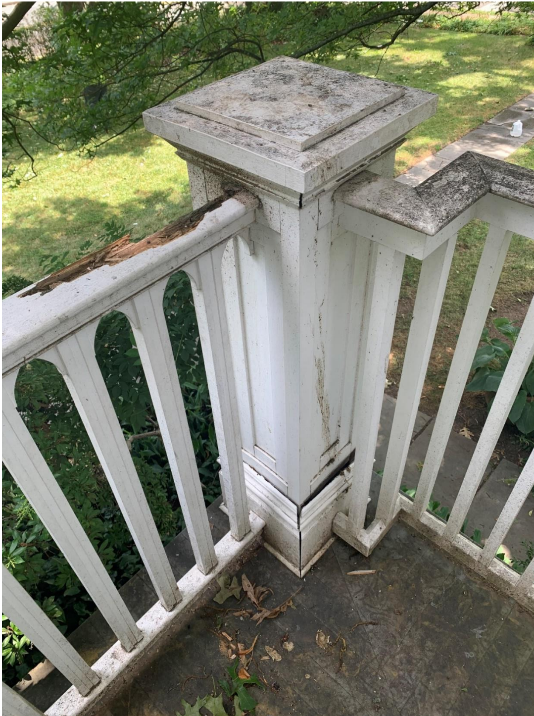
Figure 27. Damaged handrail post at porch.
