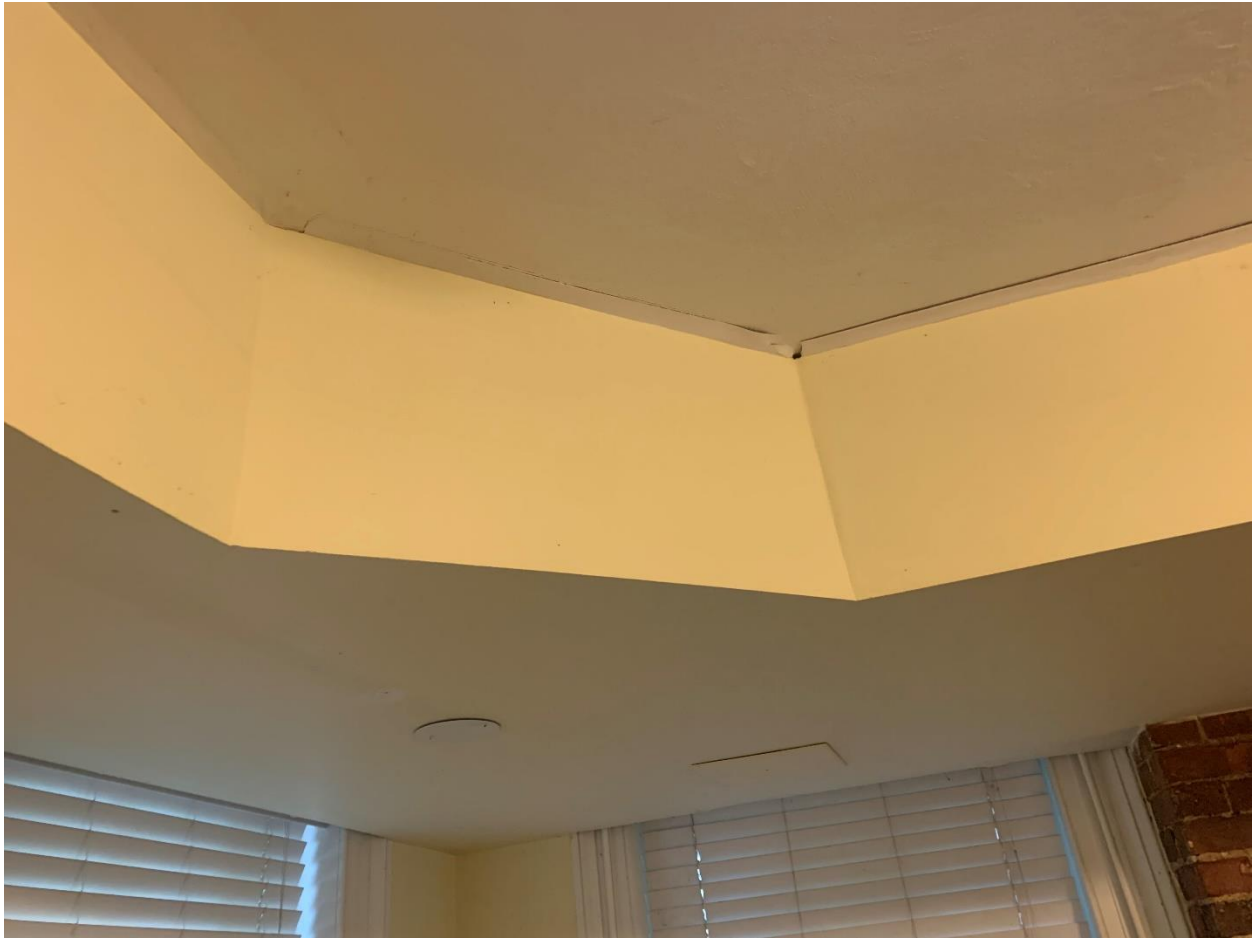
Figure 2. Basement Drywall Separation at ceiling near corner of room located at basement level.
