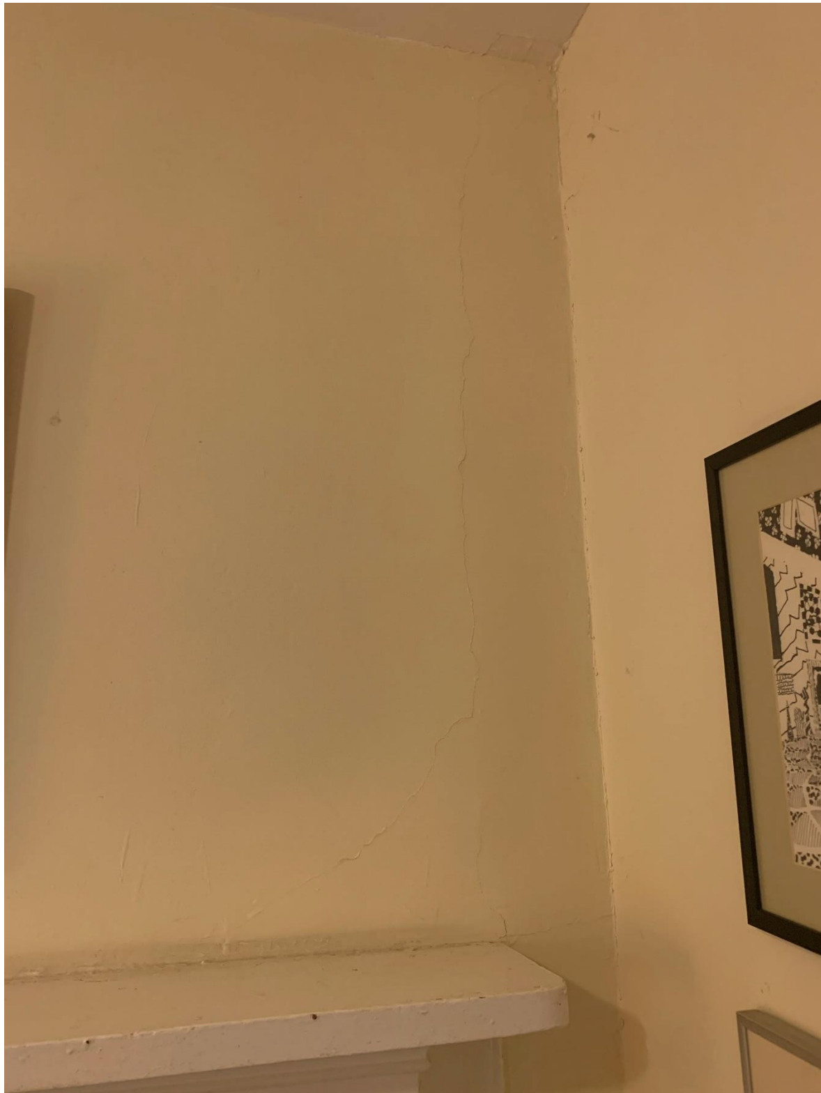
Figure 19. Suite 2B- Cracking along the wall located at the second level.
